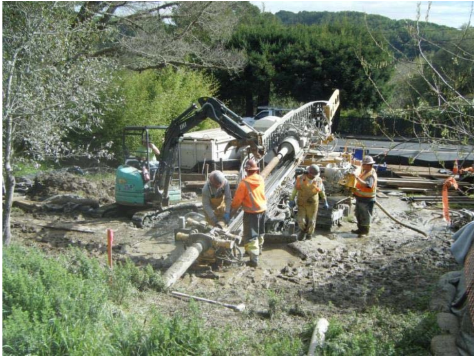
Photo 1. Drill Tech installing additional drill rods to reach a total depth of 330 feet.
