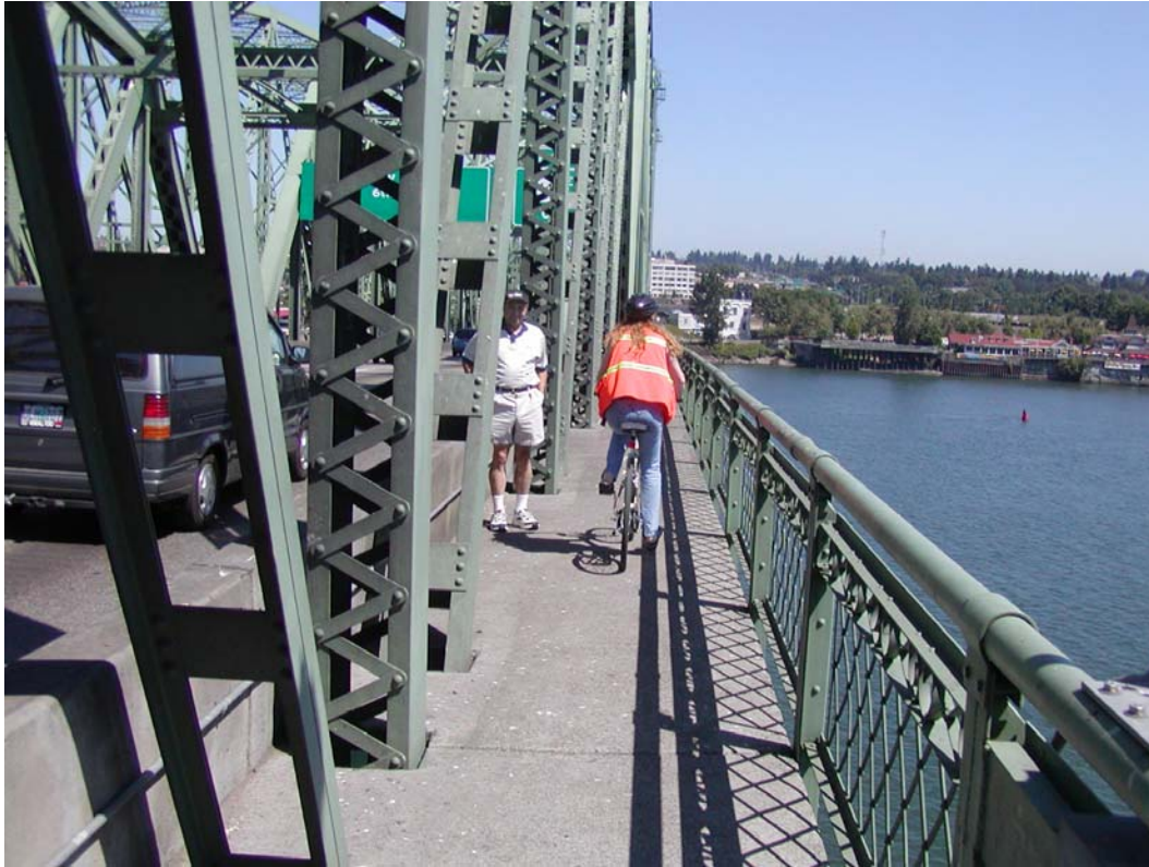
Figure 2: The pathways on the existing I-5 Bridge are four feet wide and do not meet Americans with Disability Act guidelines.
